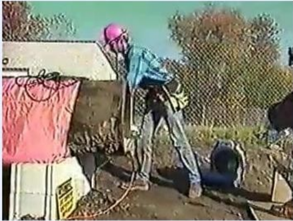
Worker in a pink hard hat and safety harness standing near a confined space entrance, holding a communication line.
