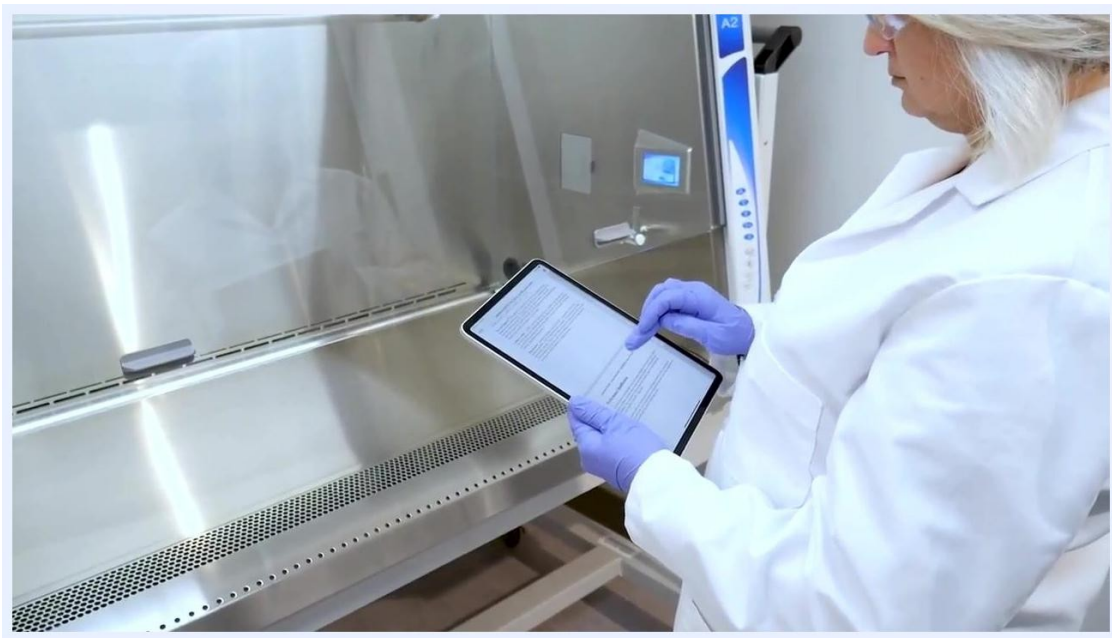
A Class II biosafety cabinet installed in a laboratory corner with clear space around it and no obstructions.
