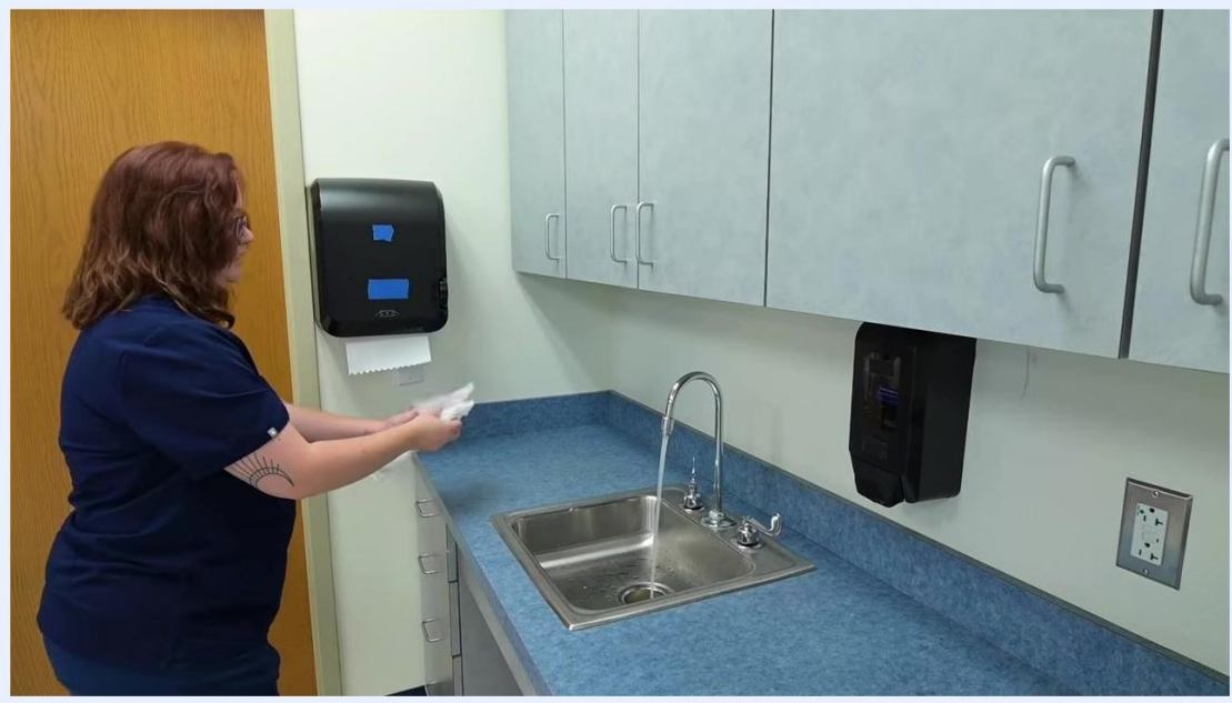
A nurse retrieves a paper towel from the dispenser in preparation for drying hands at the clinical sink, with the sink, faucet, and dispensers visible.
