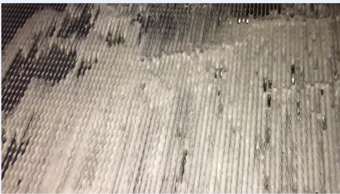
Hand brushing the foamed evaporator coil with a plastic brush
