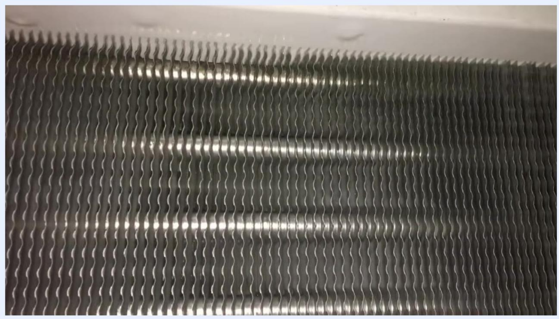
Close-up of evaporator coil fins showing a clean surface with minor spots and a uniform wavy pattern
