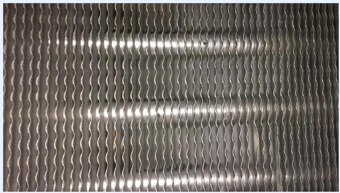
Close-up of clean HVAC coil fins with bright reflections indicating a well-maintained surface
