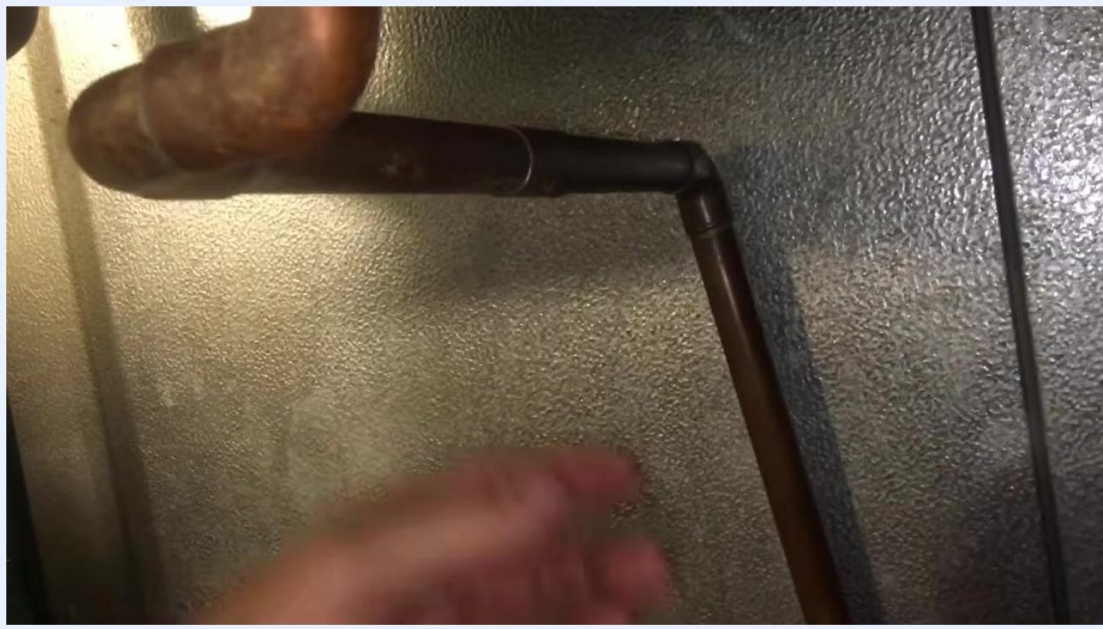
Wide view of the copper drain line running along the wall, with food storage containers below
