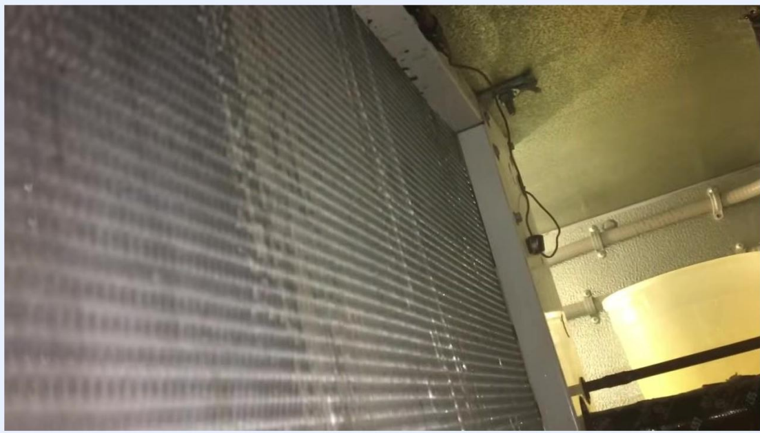
HVAC coil, white frame, and mechanical room piping, emphasizing direct hot water application
