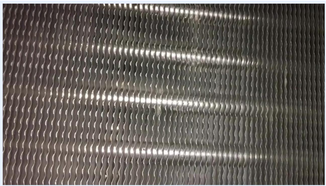
Close-up of evaporator coil showing a mostly clean surface with some minor dark areas
