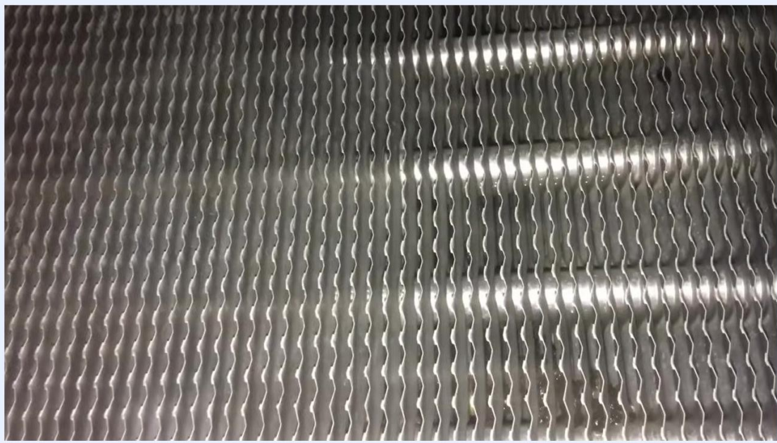
Heat exchanger tubes with visible water droplets from recent cleaning
