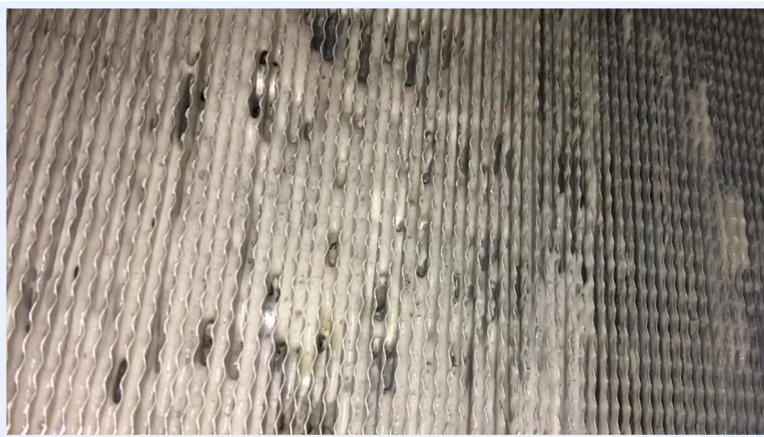
Evaporator coil fins with foaming cleaner breaking down grime after several minutes
