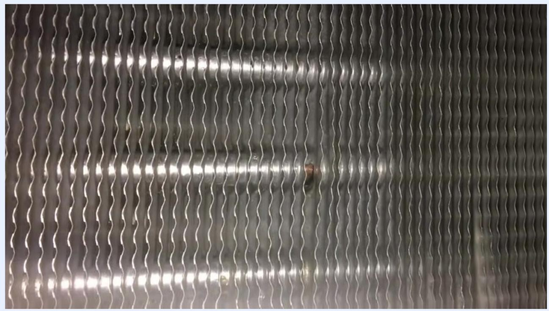
Close-up of evaporator coil fins showing a clean, metallic surface with uniform wavy patterns
