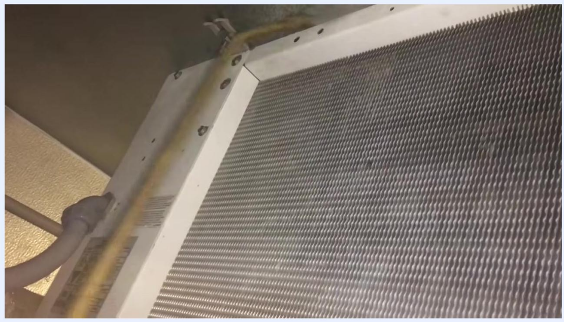
Close-up of HVAC coil, white metal frame, mounting screws, and copper pipe during thorough rinsing
