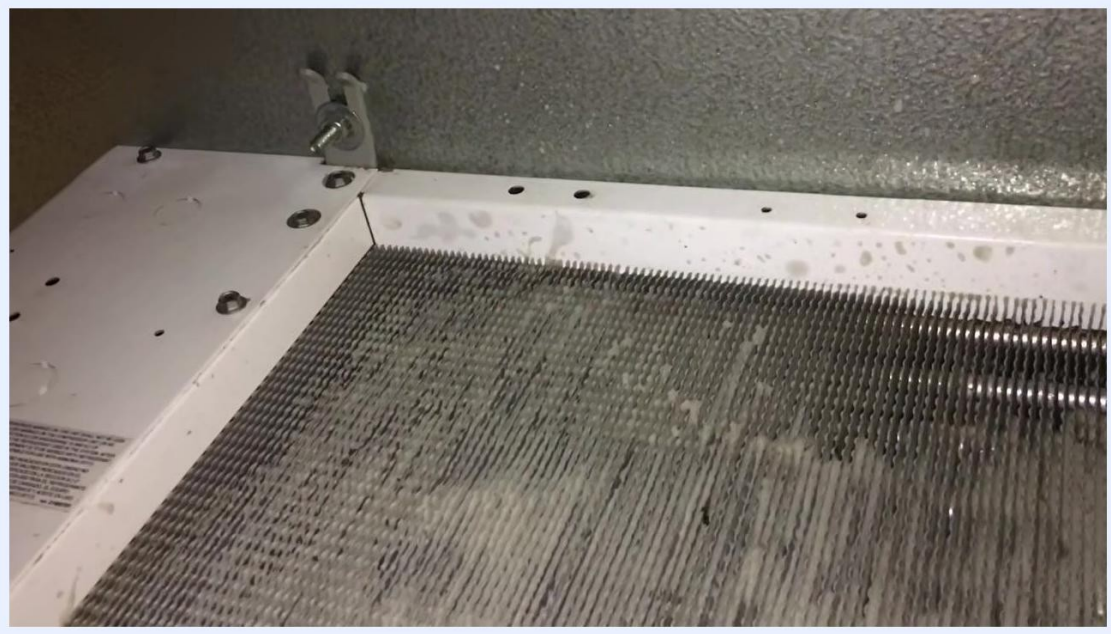
Water spray directed at the coil, with a nozzle in use
