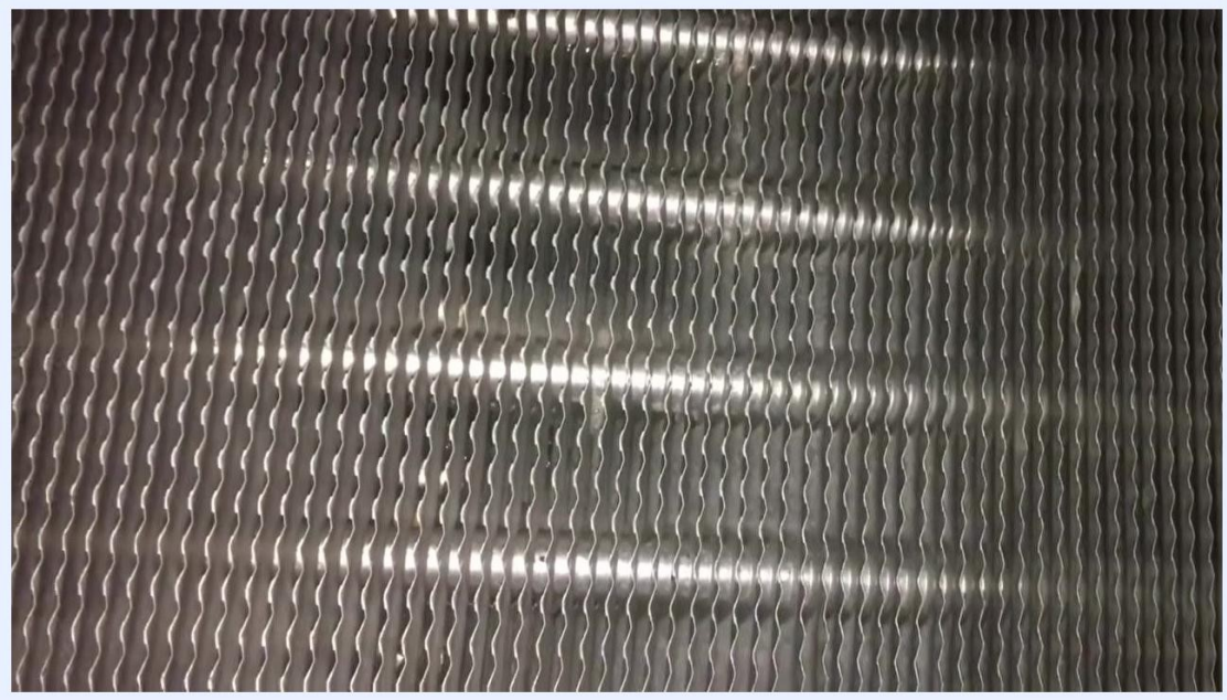
Close-up of evaporator coil fins showing a clean, metallic surface with bright reflections
