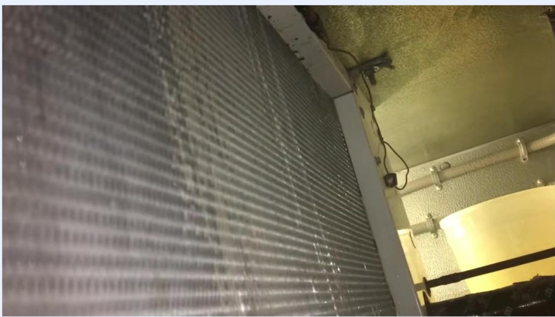
Close-up of the HVAC coil, sprayer wand tip, yellow bucket, and pipes in the mechanical room
