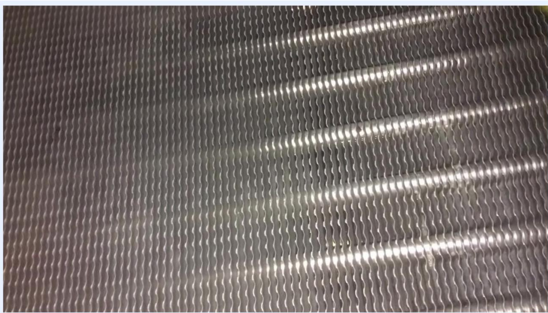
Heat exchanger tubes, clean and metallic, with some water droplets visible
