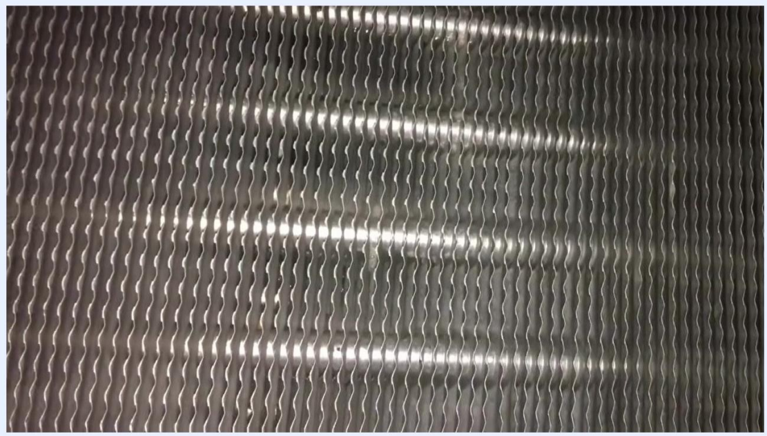
Close-up of evaporator coil with visible dark spots or residue between the fins
