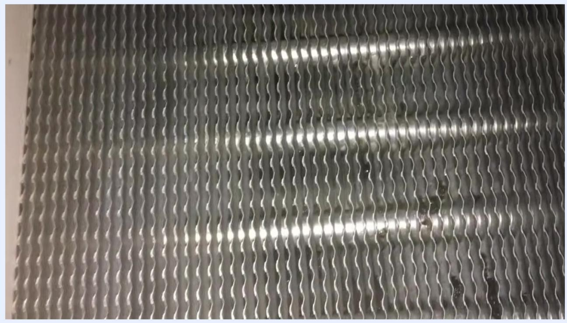
Close-up of the upper left corner of the evaporator coil showing clean metallic fins and a mounting screw
