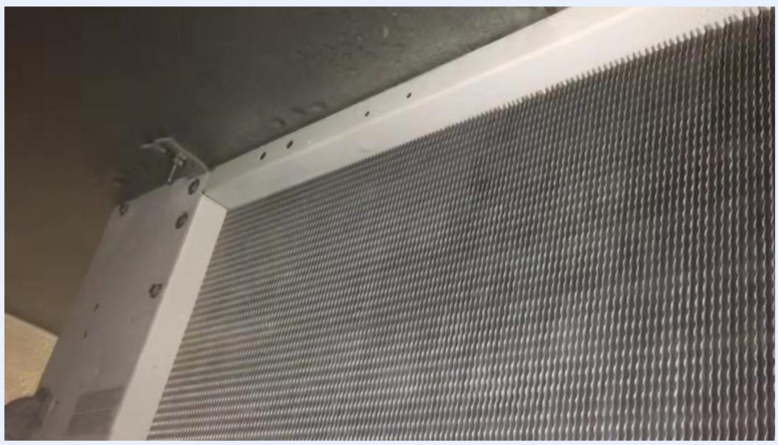
Close-up of clean HVAC coil fins and white frame
