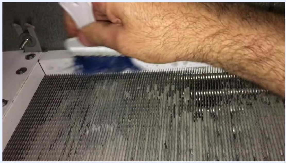
Hand brushing the evaporator coil in an up-and-down motion
