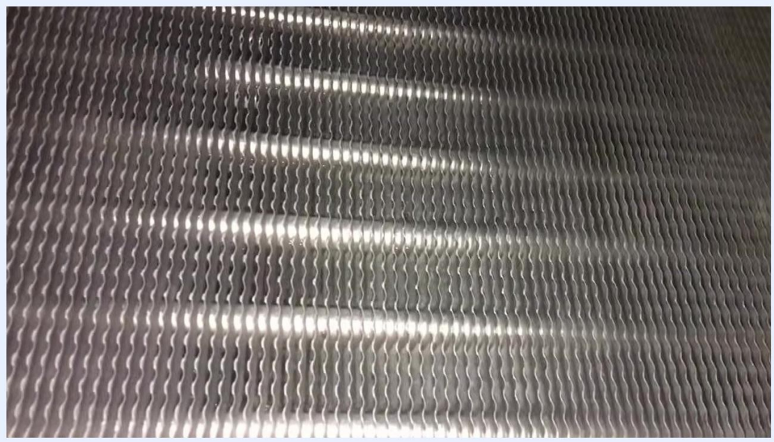
Final close-up of the evaporator coil showing a clean, metallic, and uniform surface with no visible debris
