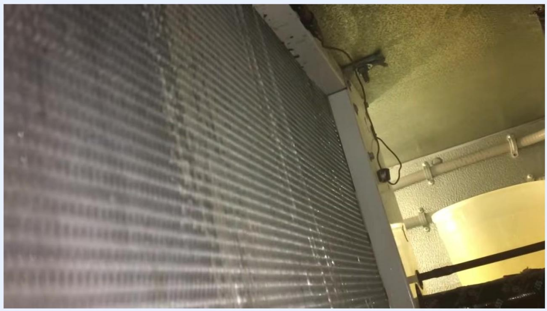
HVAC coil, white frame, and visible wiring and pipes, highlighting the need for durable hoses
