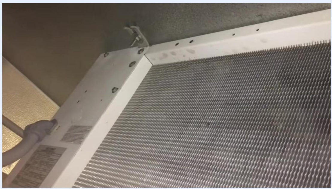
HVAC coil and mechanical room ceiling, reinforcing the importance of hot-water-rated hoses
