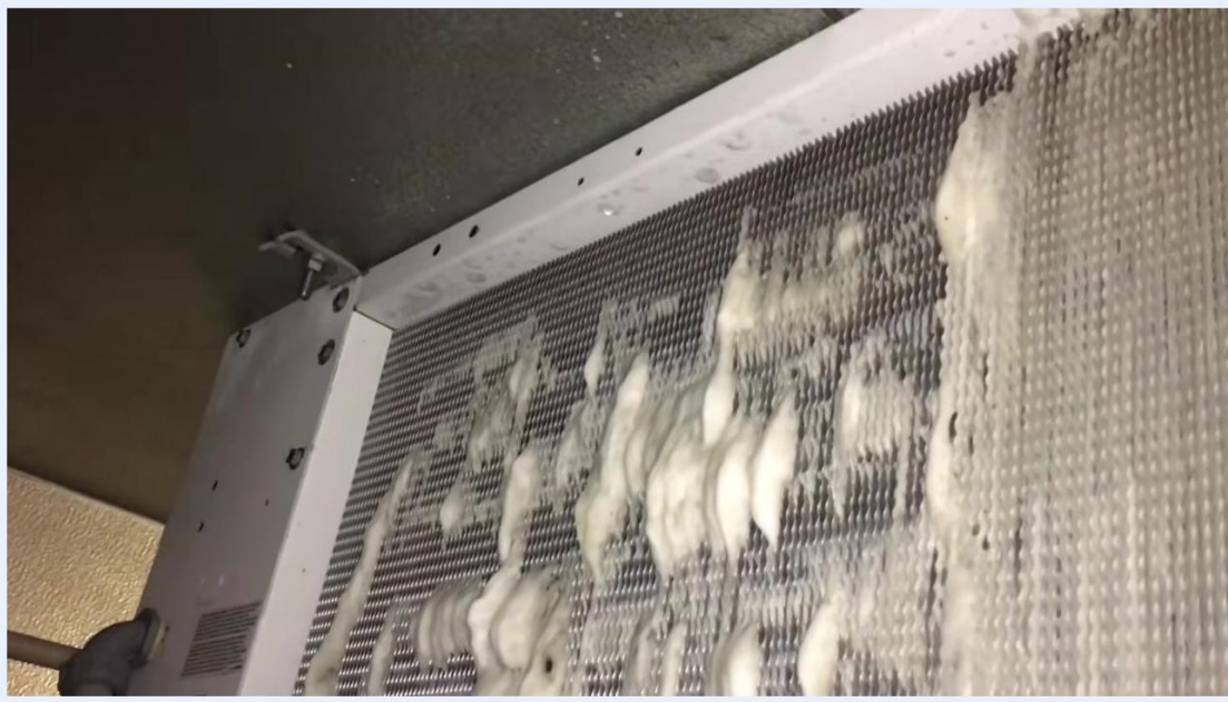
Upper right corner of the evaporator showing the temperature sensor and copper tubing
