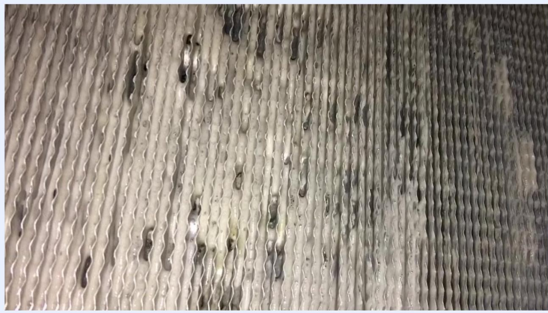
Evaporator coil fins after brushing, showing cleaner residue and improved cleanliness
