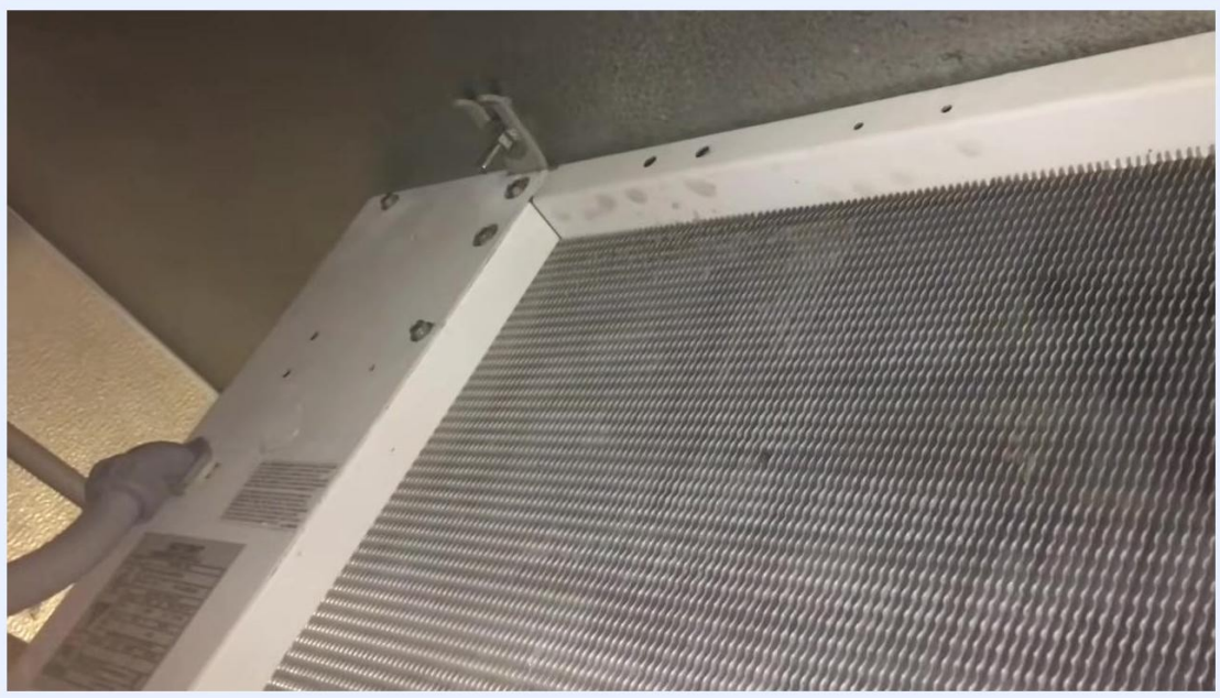
Angle of HVAC coil showing white metal frame, mounting screws, and attached pipes
