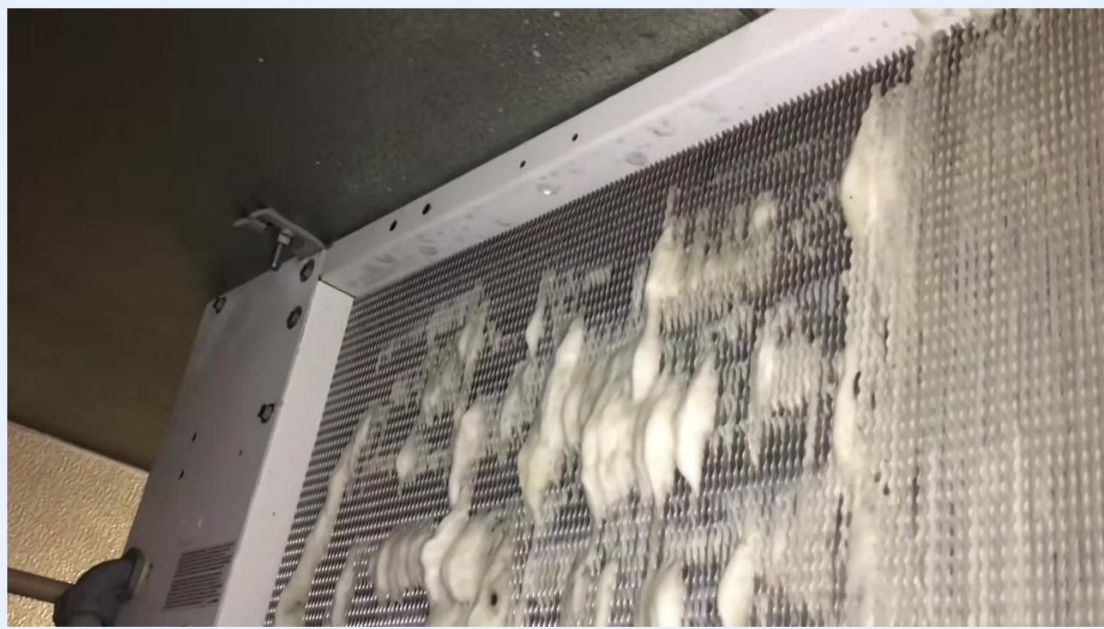
Close-up of the evaporator coil with foaming cleaner applied, showing dirt and buildup on the fins
