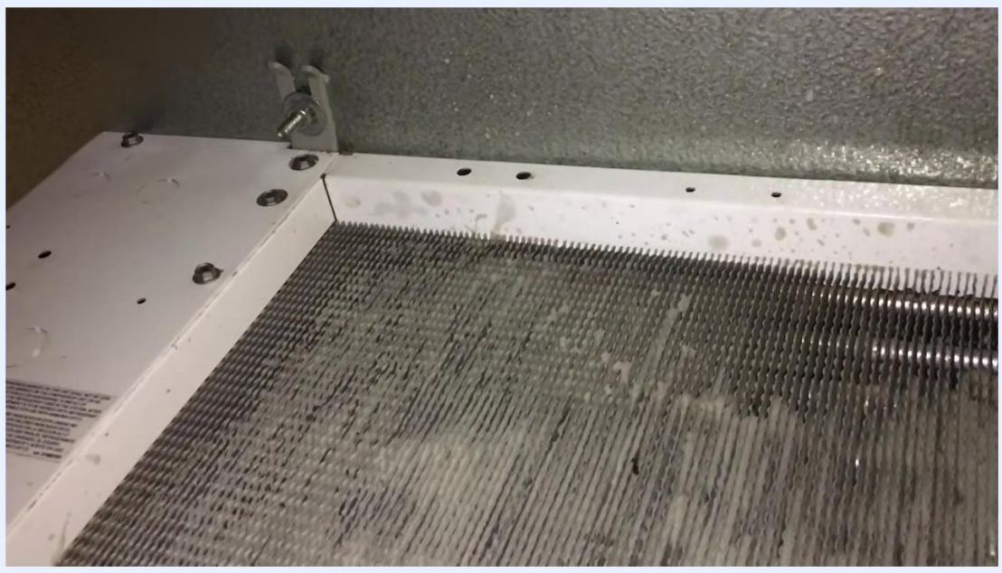
Close-up of HVAC coil and metal frame showing water spots and residue before cleaning
