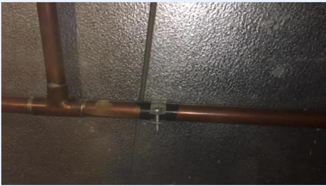
Another view of copper pipes and wall showing the workspace environment
