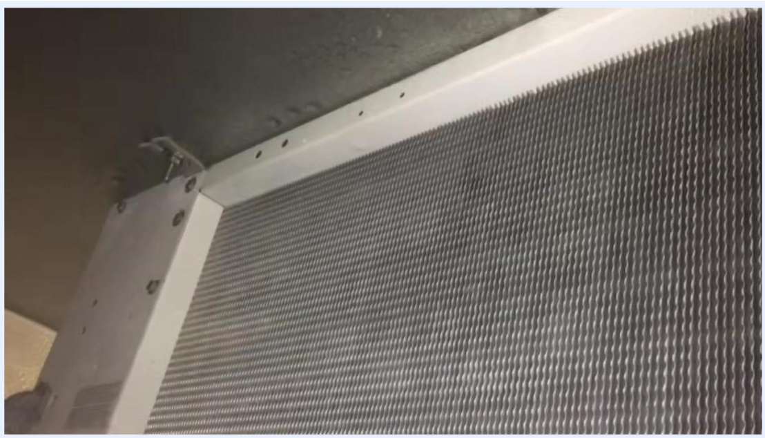
Detailed view of clean HVAC coil fins, unobstructed and free of buildup
