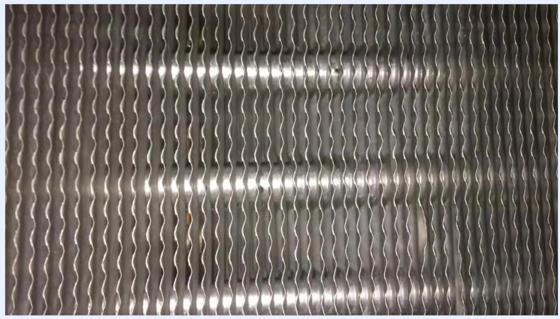
HVAC coil and white frame viewed from a different angle
