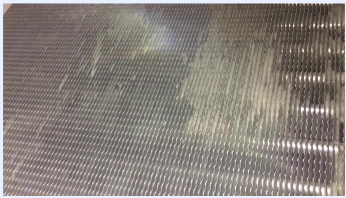
Wider view of the coil and surrounding area, including pipes and wall
