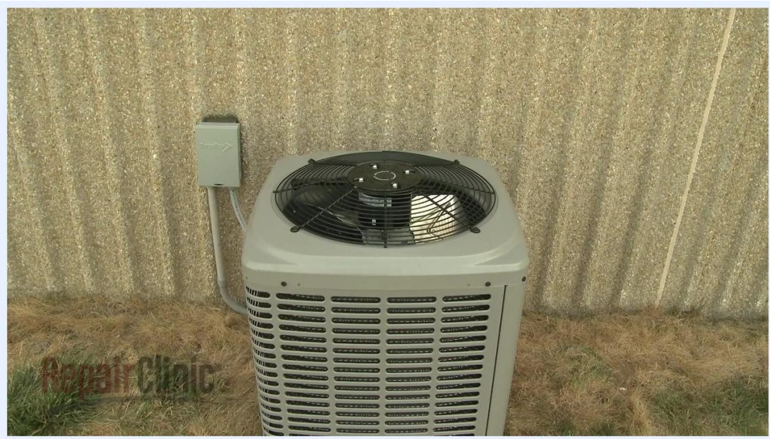
Outdoor central air conditioning unit next to a wall, a typical location for a capacitor
