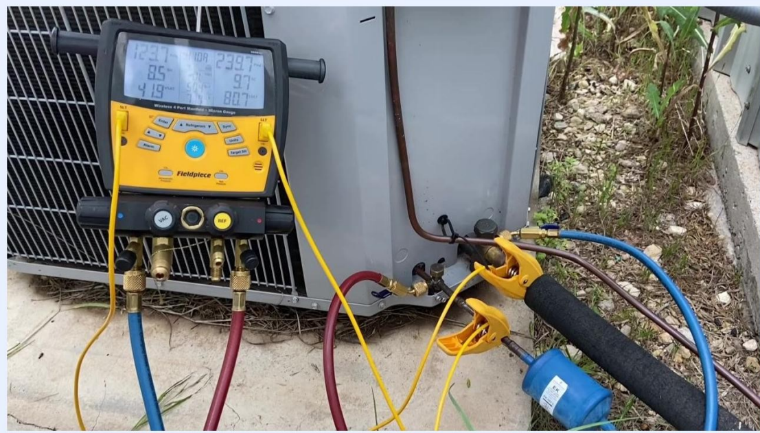
Fieldpiece digital manifold gauge connected to an outdoor AC unit, displaying live superheat and subcooling values. Hoses and temperature clamps remain attached, with the unit positioned outdoors on gravel near vegetation.
