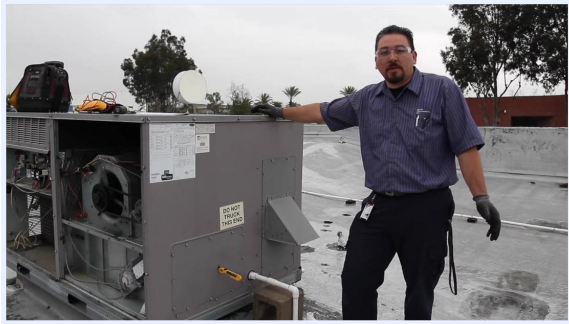
Technician standing next to the HVAC unit on a rooftop with the access panels open, explaining the economizer function and inspection.
