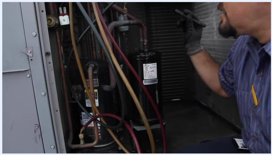
Technician referencing the compressor and electrical connections, preparing to check amp draws.
