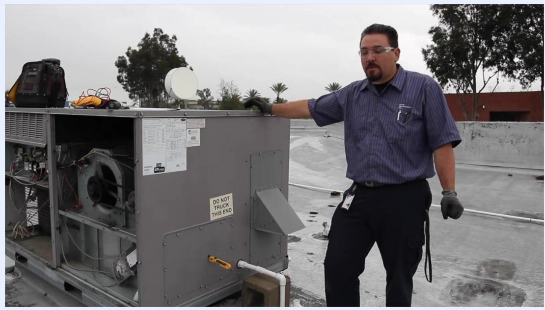
Technician standing next to an open rooftop HVAC unit, with tools and warning labels visible.
