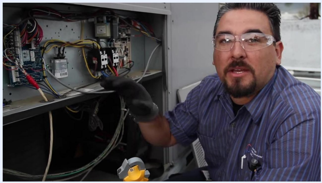
Technician explaining the need to replace the capacitor, holding a clamp meter inside the open electrical compartment.
