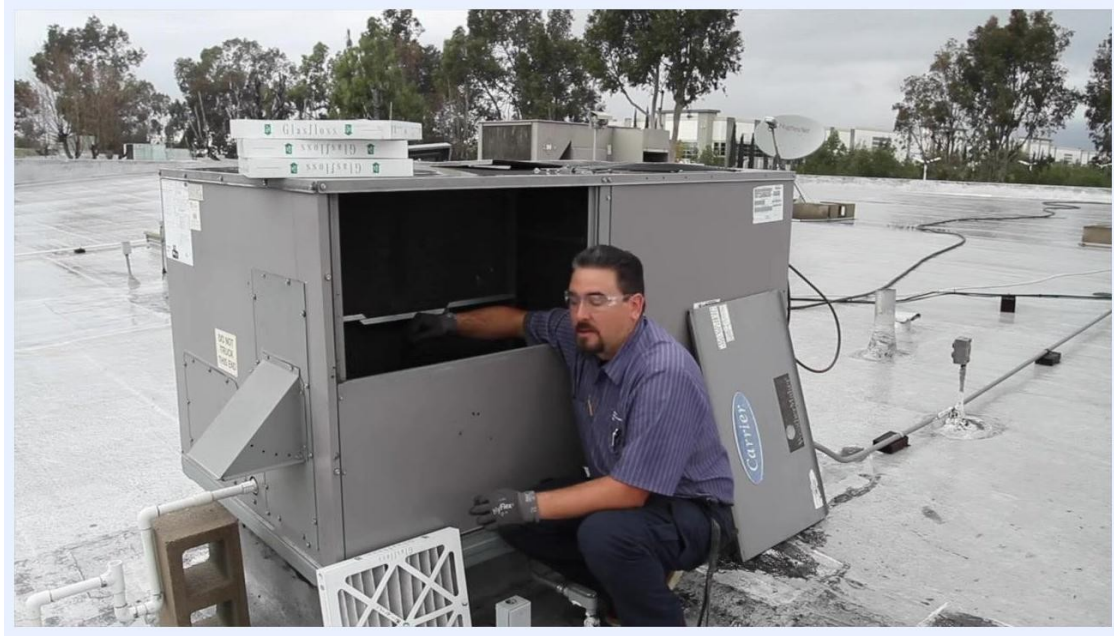
Technician reaching inside the HVAC unit to check or clean the drain pan.
