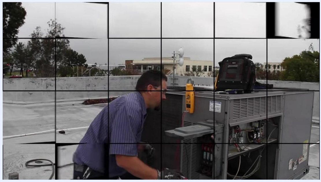
Technician standing next to an HVAC unit on a rooftop with a multimeter and tool bag on the unit; the access panel is open, exposing internal components.
