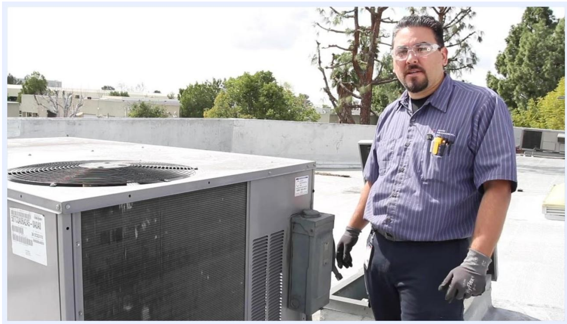
Technician standing next to a rooftop HVAC unit with one hand near the electrical disconnect box, preparing to restore power.
