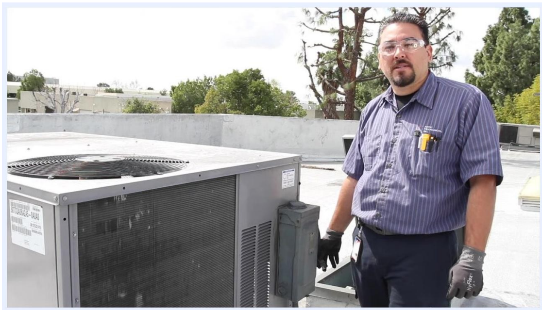
Technician standing beside the HVAC unit, addressing the camera, wearing safety glasses and gloves, with company branding visible on the shirt.
