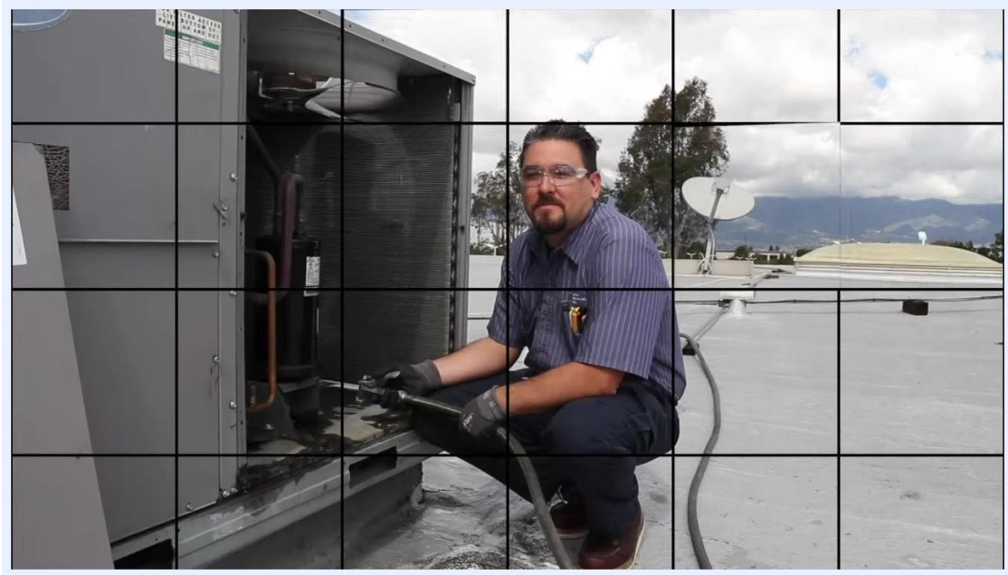
Technician kneeling by the open HVAC unit, pointing to the fuse compartment with the multimeter hanging nearby.
