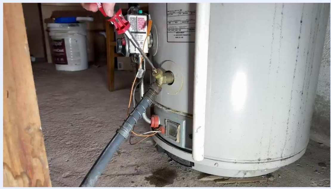
Rust-colored water and sediment draining from a hose into a floor drain.
