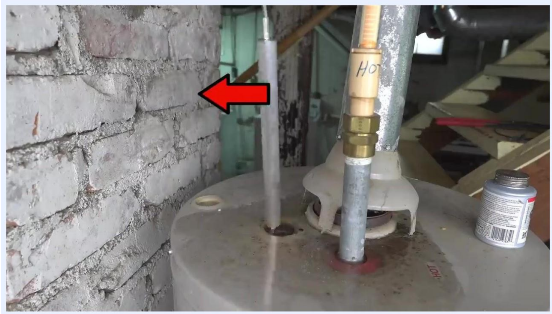
A water heater with the anode rod removed, next to a pipe labeled "HOT," with a red arrow pointing to the anode rod opening.
