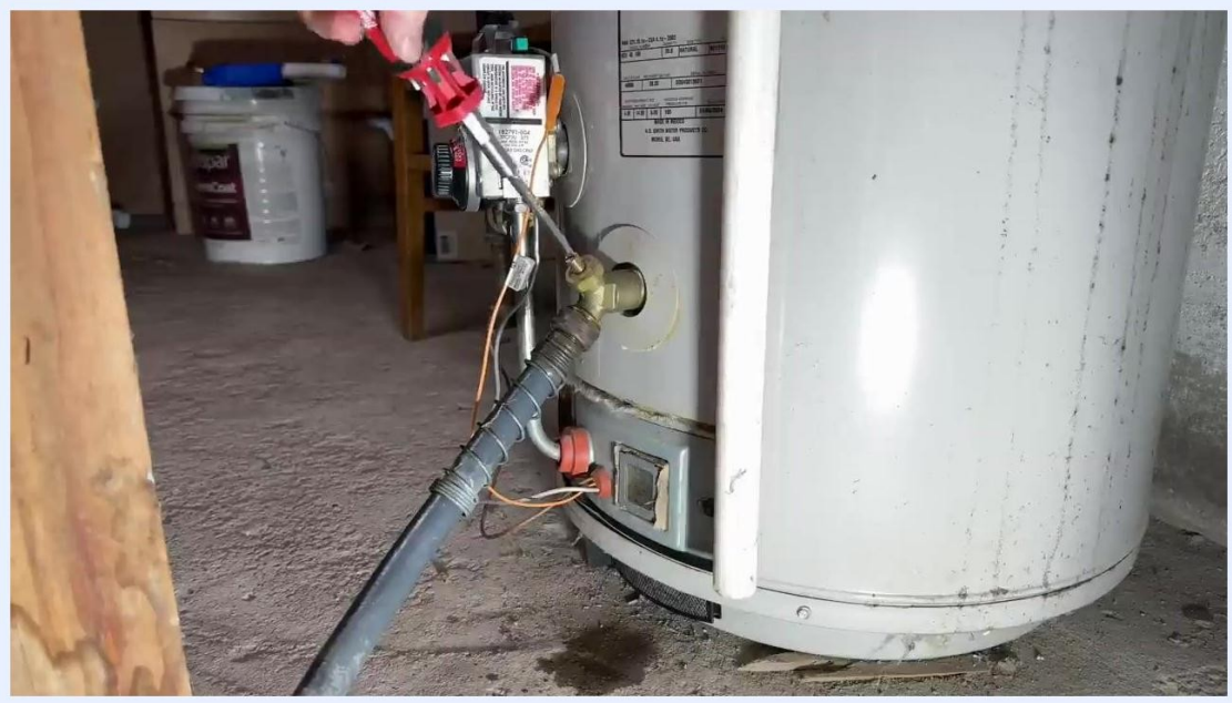
A hand operating a blue valve on a pipe, with an inset image showing brown water draining into a clear container.
