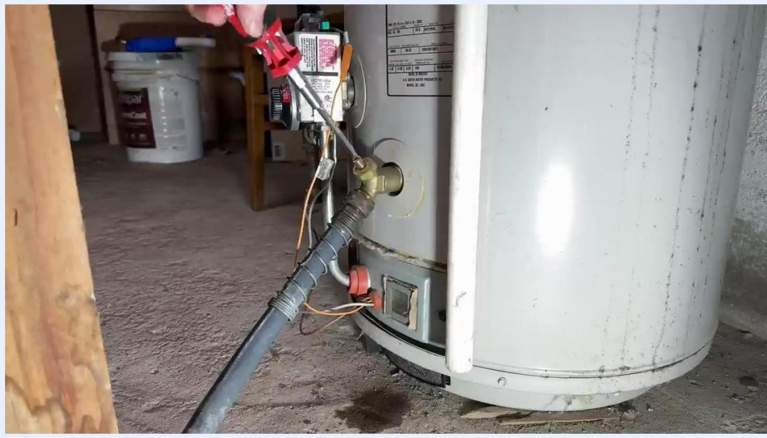
Close-up of a garden hose connected to the water heater's drain valve, being opened with a screwdriver.
