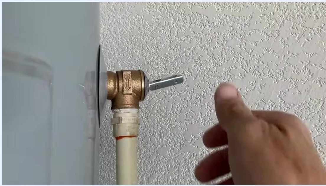
Hand reaching to close the brass drain valve on the water heater
