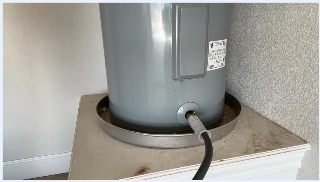
Garden hose securely attached to the water heater drain valve, ready for draining
