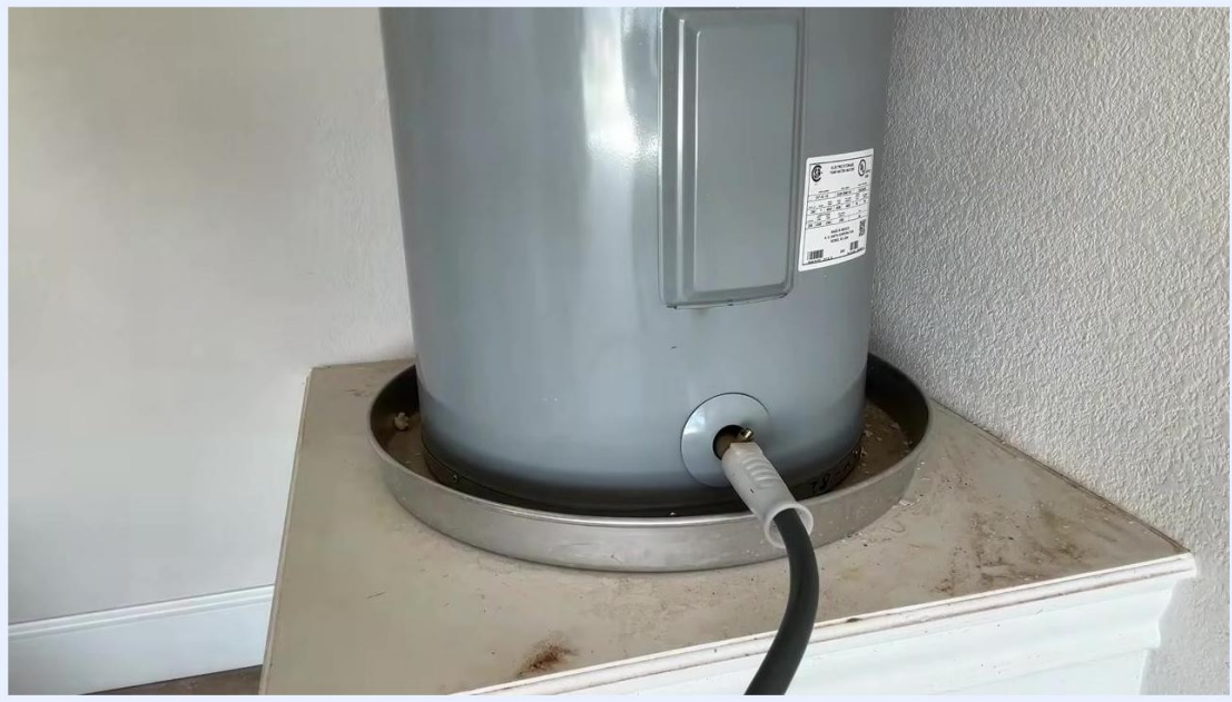
Person next to a water heater, preparing to shut off the cold water supply valve
