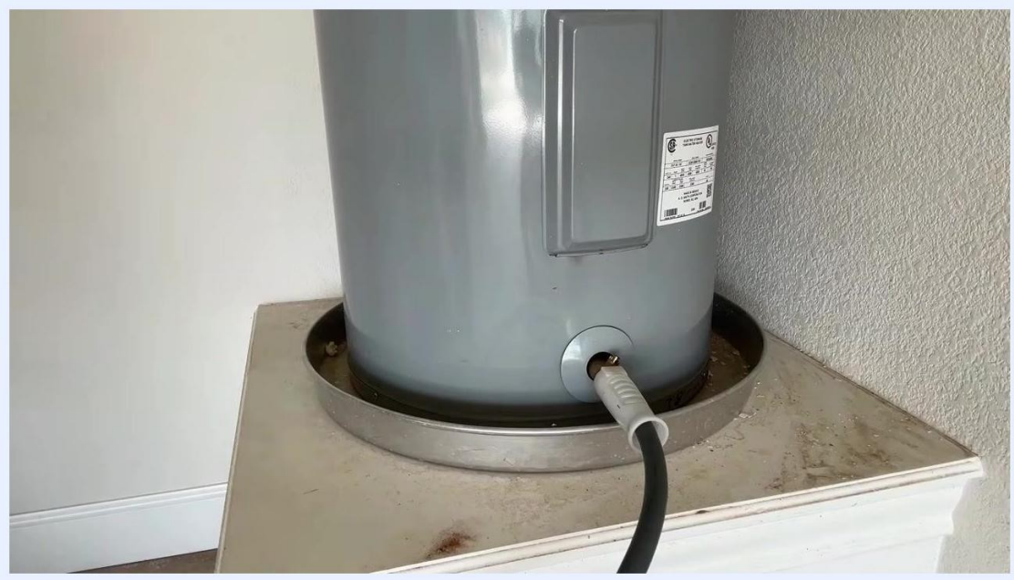
Water heater with hose attached and water draining, no person visible
