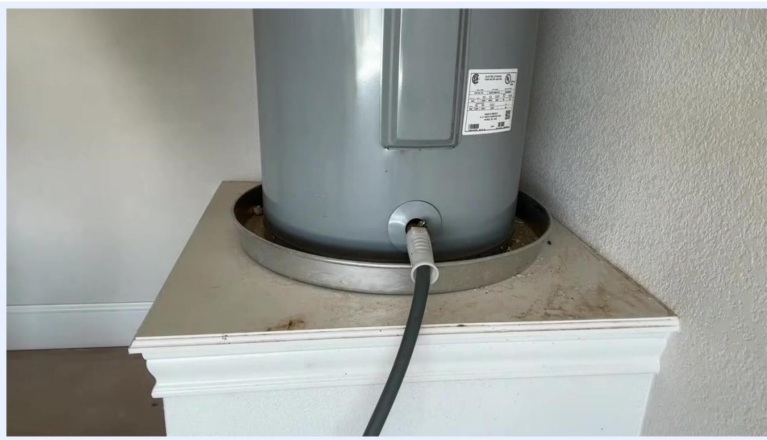
Water heater with hose attached, draining after a repeated flush, no person visible
