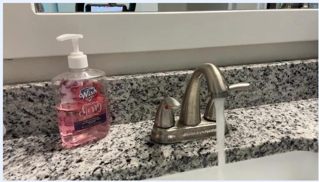
Hot water faucet running in a bathroom, bottle of Wish Ultra hand sanitizer visible
