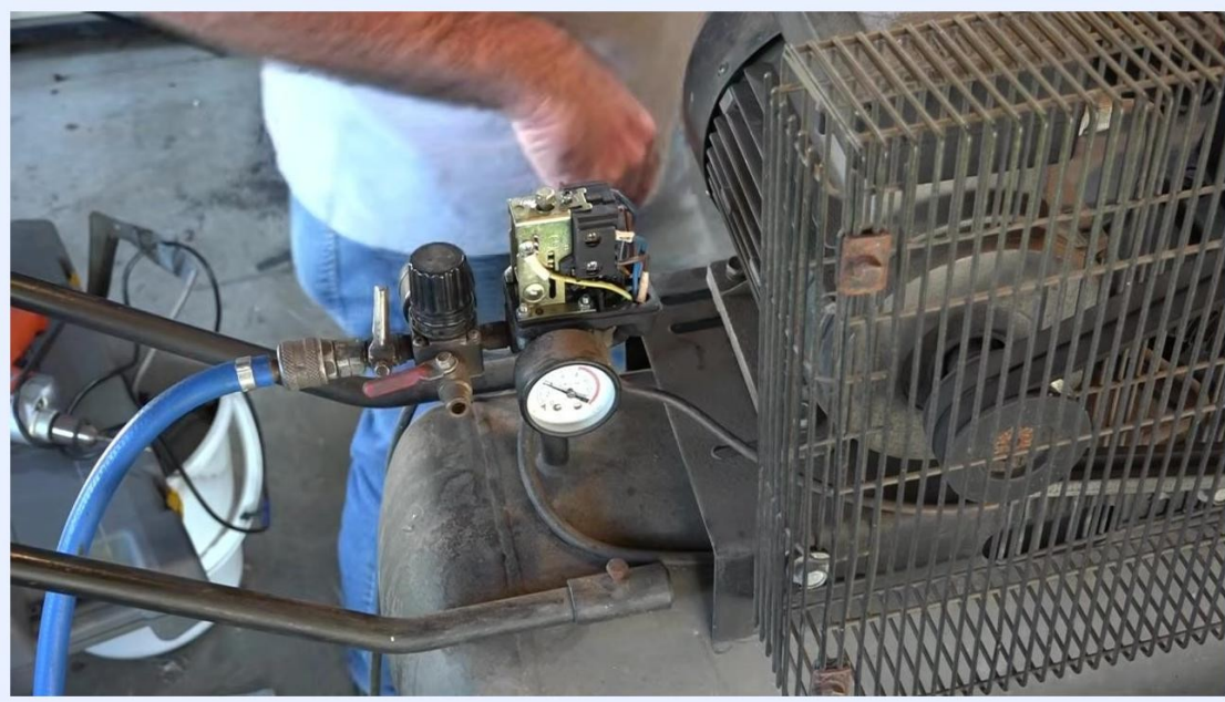
Air compressor with an exposed pressure switch, pressure gauge, regulator, and blue air hose in a workshop with tools in the background
