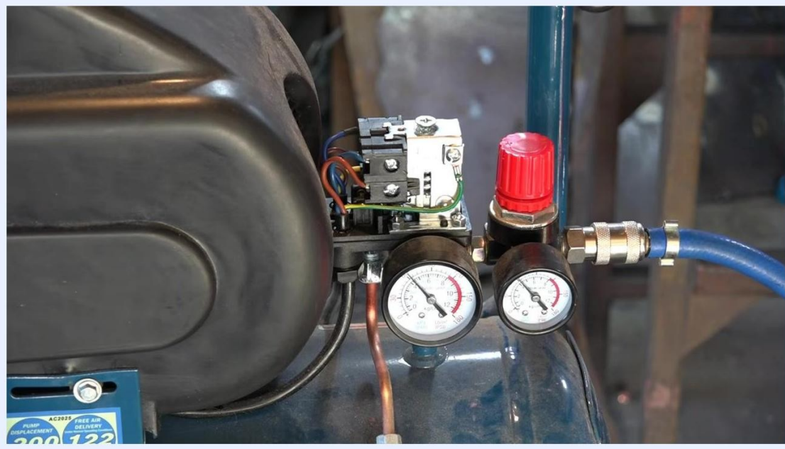
Compressor gauges showing the lowest pressure setting achieved after adjustment
