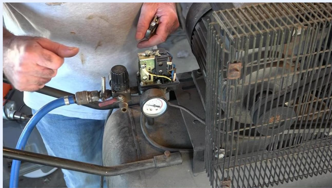
Pressure gauge on the compressor tank showing just over 50 psi, with the pressure switch exposed and the adjustment complete
