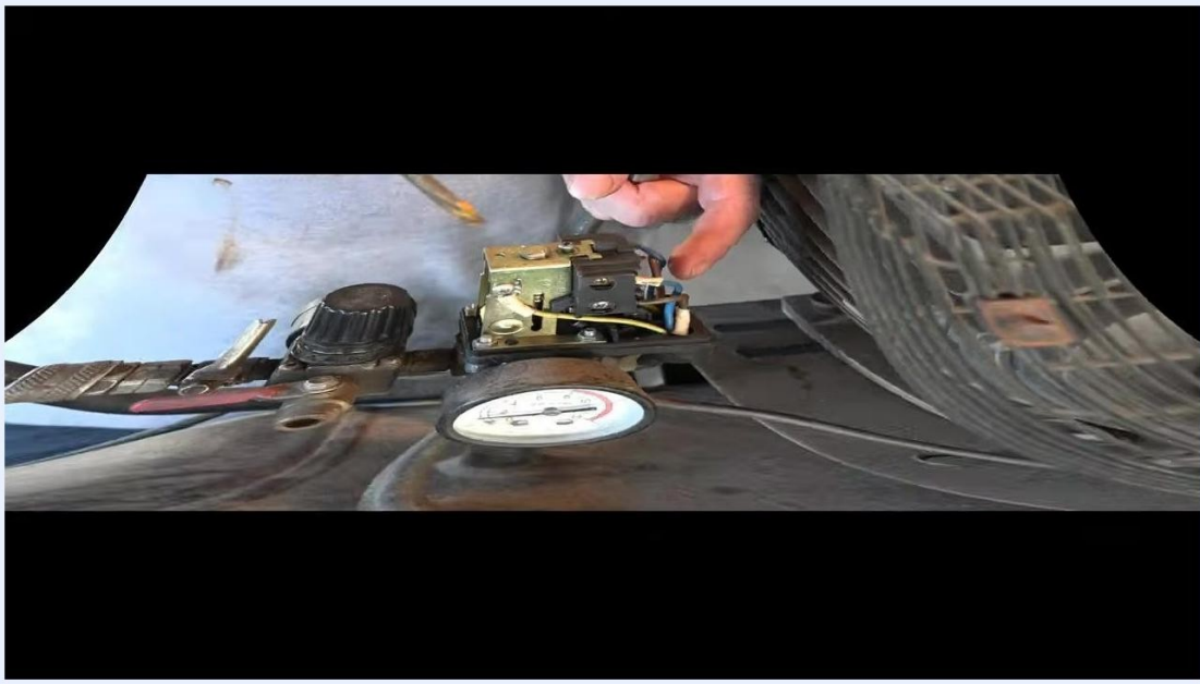
Pressure switch cover removed, exposing internal components including adjustment screws, wiring, and a metal plate
