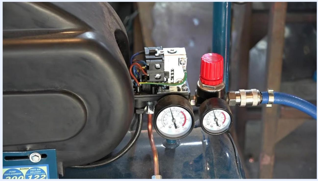
Close-up of compressor gauges showing tank pressure just under 90 psi, with the red regulator knob and wiring visible
