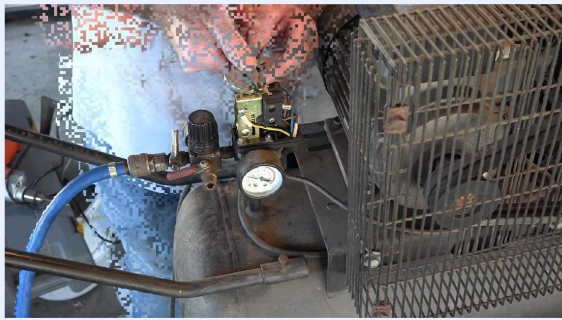
Hand using a wrench to adjust the top screw on the pressure switch, lowering the cut-off pressure, with the gauge and wiring visible
