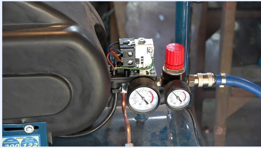
Compressor gauges and assembly with pressure stabilizing after repeated air release
