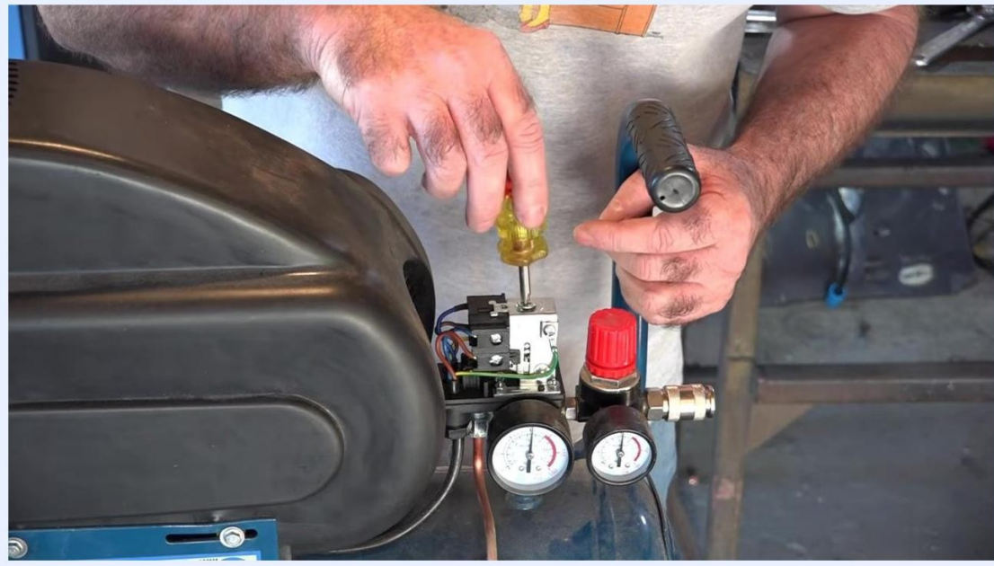
Phillips screwdriver pointing at the adjustment screw on top of the pressure switch, with dual gauges and the red regulator knob visible
